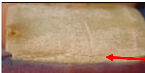
Notice the cracks in the hinge
